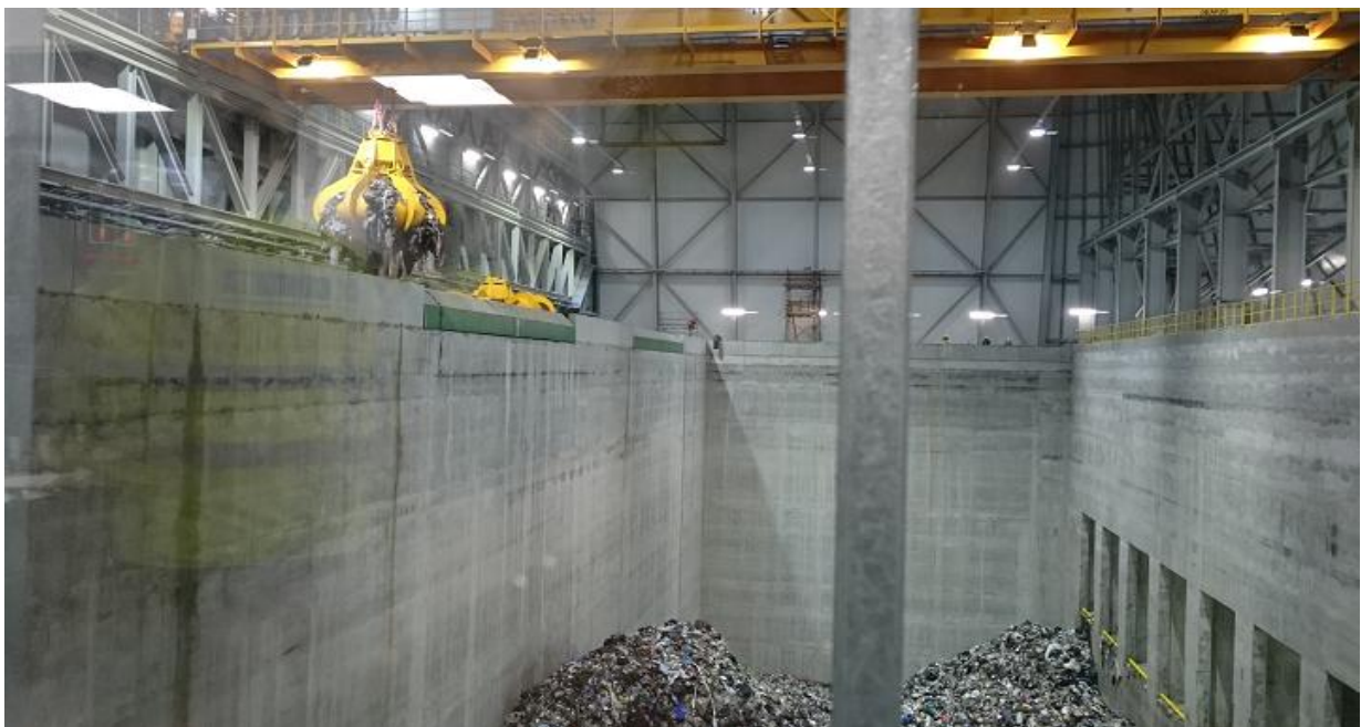
First drop of waste into feed hopper, combustion line 1 (Copyright PML).
