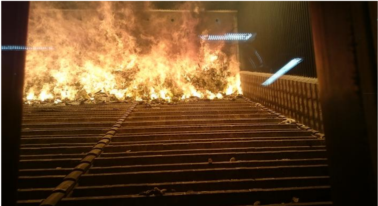
First combustion of waste on Line 1, viewed from the boiler's viewport (Copyright PML)
